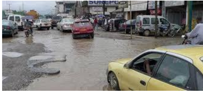
Figure 6. Road condition in coastal region
