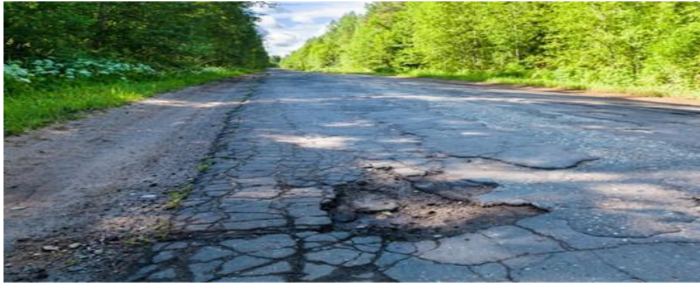
Figure 7. Road condition in coastal region
